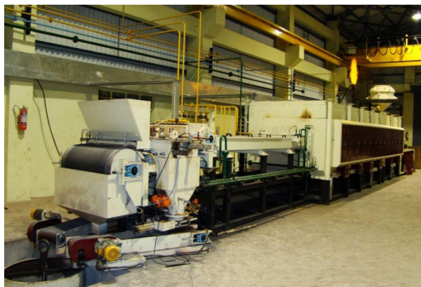
Fig. 4. Gas-tight conveyor furnace. Design of Gas Institute of NAS of Ukraine. Pilot plant for production of iron powder (300 t/year). Hyderabad, India (photo – D.M. Fedorov).
